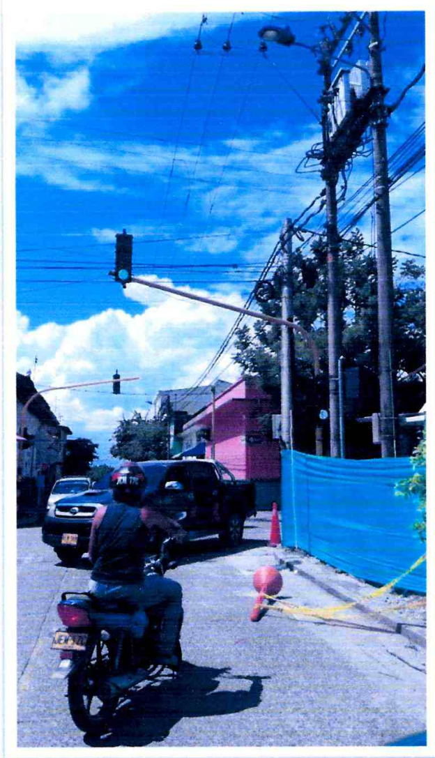
INSTALACION VEHICULAR SEMAFORO S2
